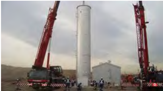
Gas collection system East Calgary Landfill
